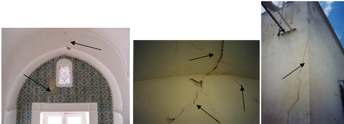
Figure 4. Initiated cracks at the corner of the building and the openings
